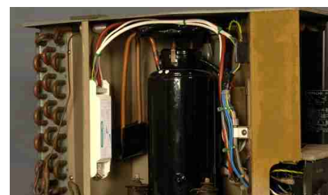
10 Check correct wiring & replace covers
