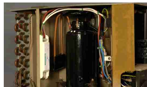
10 Check correct wiring & replace covers
