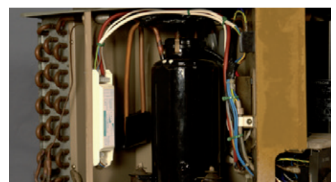
10 Check correct wiring & replace covers
